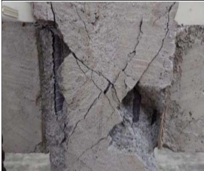
Figure 14. Collapse of Joint BJ-1
